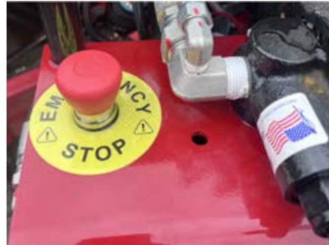
Emergency Shut Off Switch (“Panic Button”)
