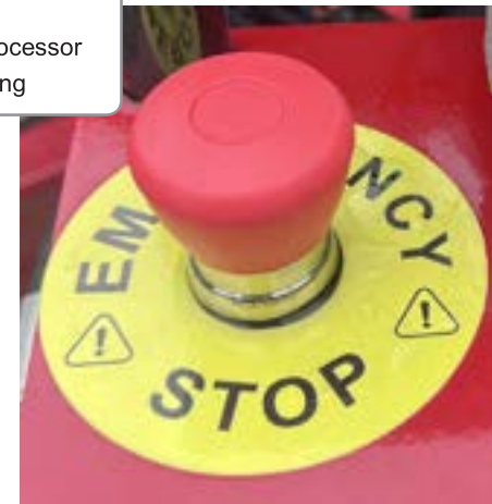
Power Plant Controls – Emergency Shut Off
